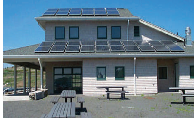
Solar panels installed by IBEW Local 103 atop the visitor's center on Spectacle Island in Boston Harbor.
